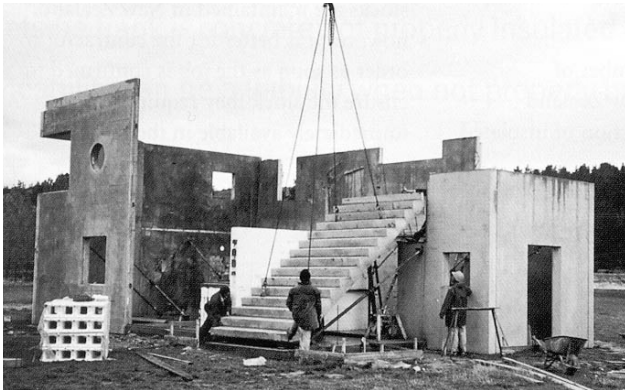
Figure 4.1 Installation of a Flight of Precast Concrete Stairs. (Image supplied by Mikael Carlstrom, Composite Systems Pty Ltd.)
